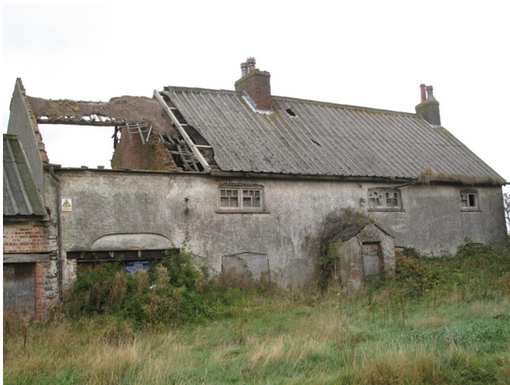
Locally listed Midgeland Farm in an advanced state of disrepair
